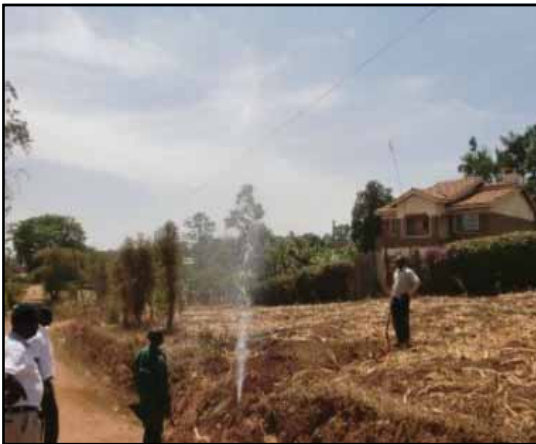
Leakage from bad connection point
